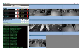
VMS-CCTV Video Management System
